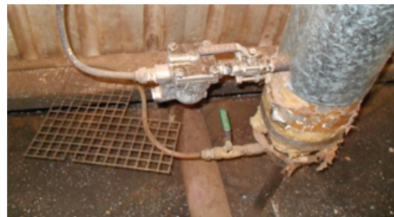
FIGURE 1 INSTALLED STEAM TRAPS
