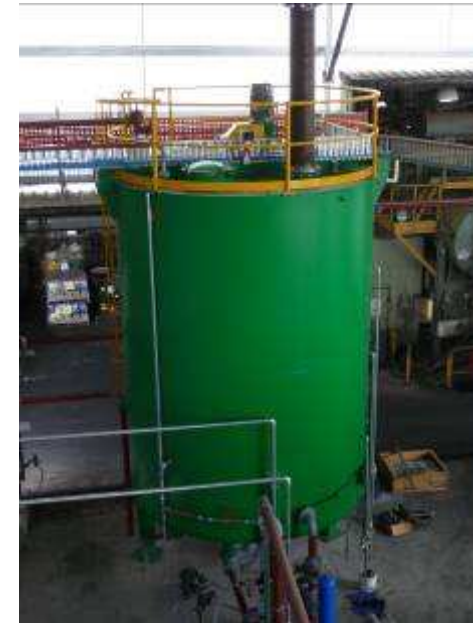
45 m3 Fuel Blending Tank
